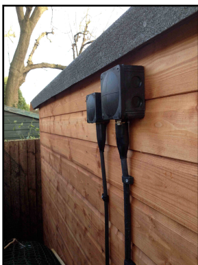
SWA cable run in steel galvanised conduit for additional protection. This can be covered safely and offers a very high level of protection against physical/rodent damage.
